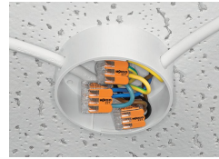
Lighting distribution in a ceiling canopy
